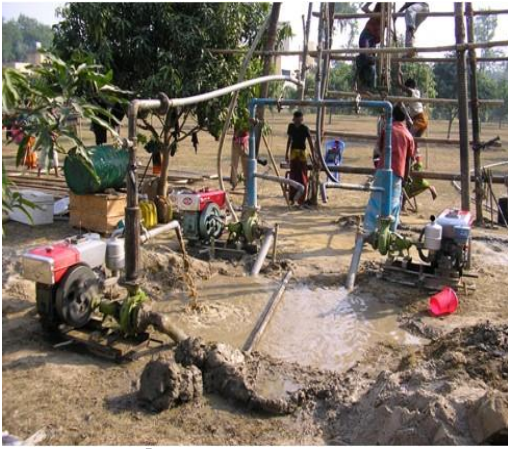
Figure : Three pumps are using as a circuit
