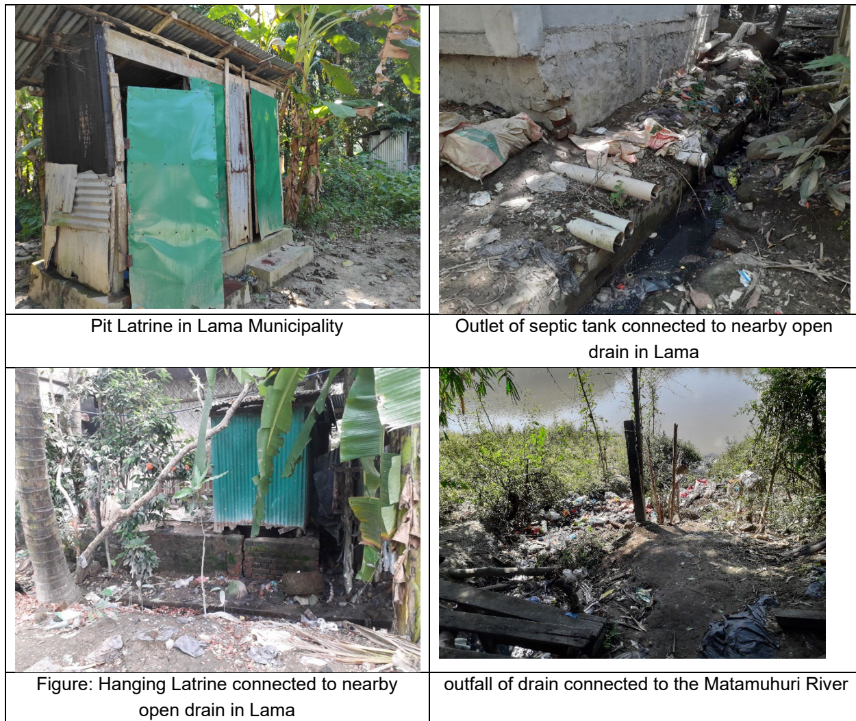
Figure 3: Photographs showing existing sanitation system
